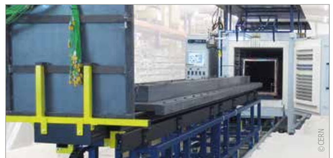
Production furnace with a special loading and unloading system.
